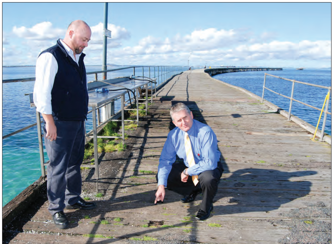
SHIRE Director of Engineering Gavin Harris and CEO Mal Osborne point out an area of concern on the Esperance Tanker Jetty.
