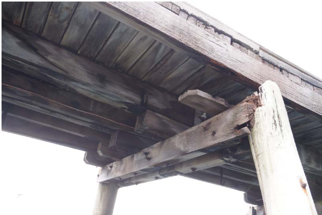
The corbel has split and fallen away and the stringer is no longer supported by the pile underneath.
