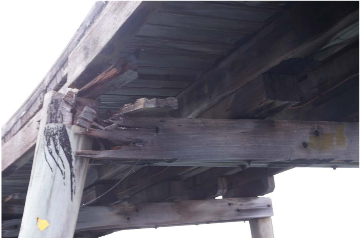
The red wood exposed is indicative of recent failure in the half cap and corbel, highlighting that the jetty is twisting and creating new damage.
