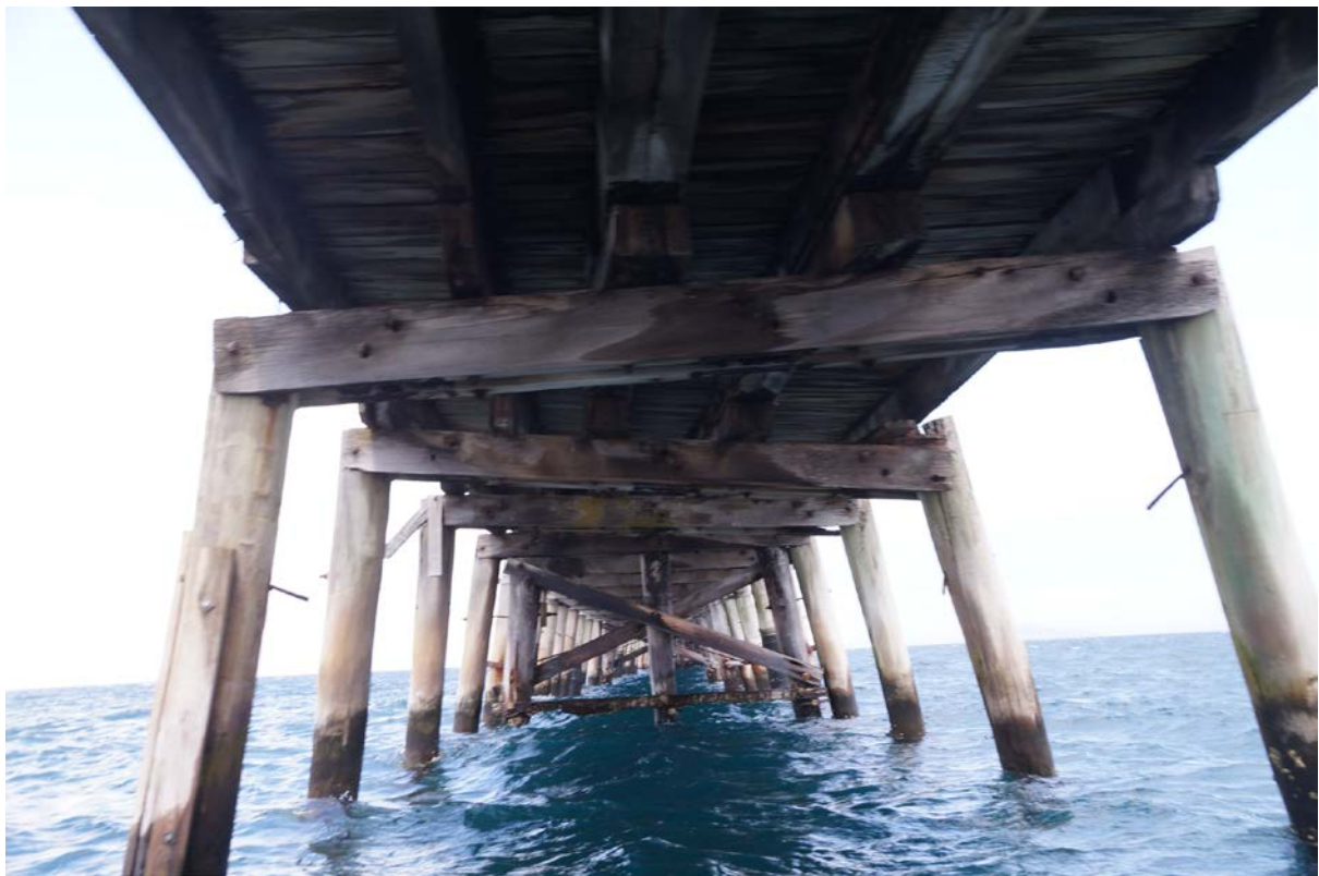
The pile on the left hand side, which already has a splint applied from previous repairs has completely failed and is no longer supporting the deck. The half cap at the front of the photo has collapsed to the north and the next two half caps have collapsed to the south, making the deck twist.
