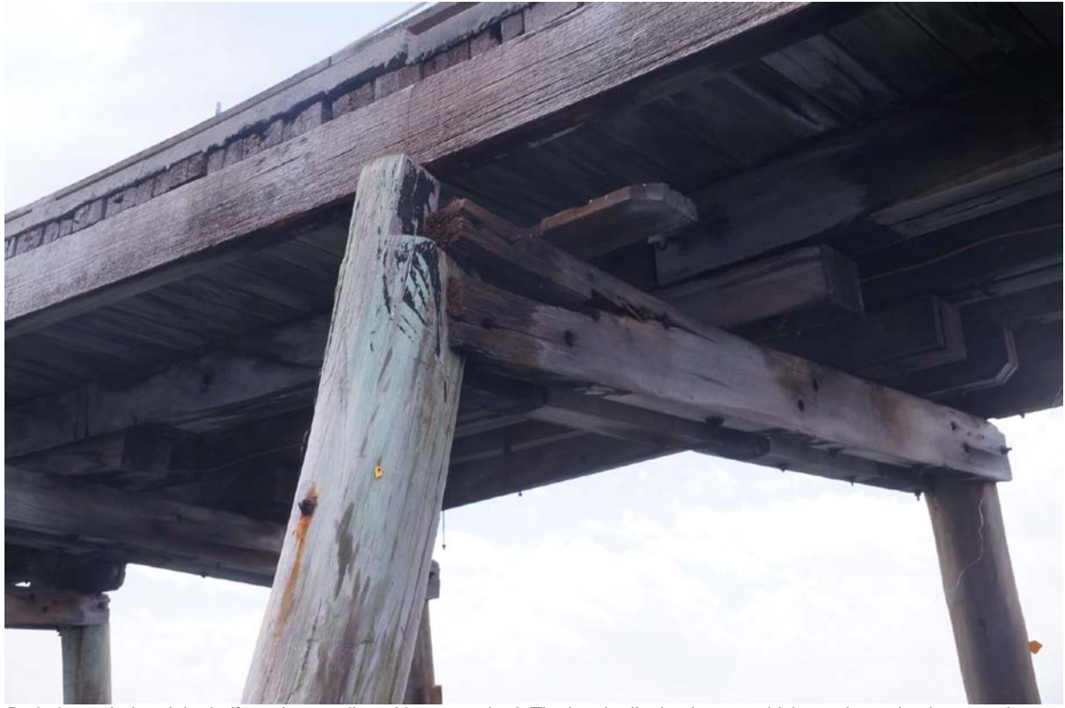
Both the corbel and the half cap have split and been crushed. The longitudinal stringers, which are the main elements that support the deck are no longer supported by the half cap. This damage has accelerated since December 2015 and is causing the deck to sag.
