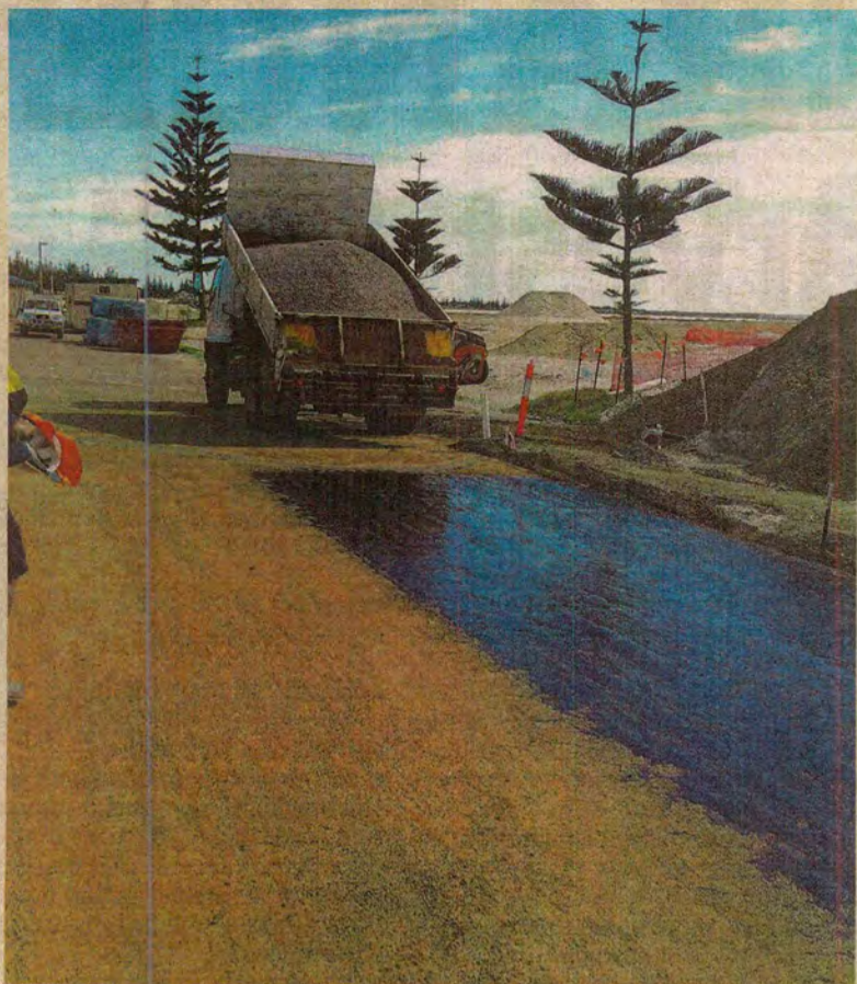
Extended carpark: Spray seal is applied to the extended carpark near the tanker jetty, which should re-open this week. Photo: SHIRE OF ESPERANCE
