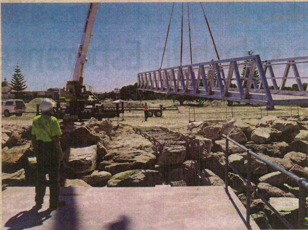
Bridging gap: Workmen place the aluminium onto the tanker jetty last week. Photo courtesy: SHIRE OF ESPERANCE
