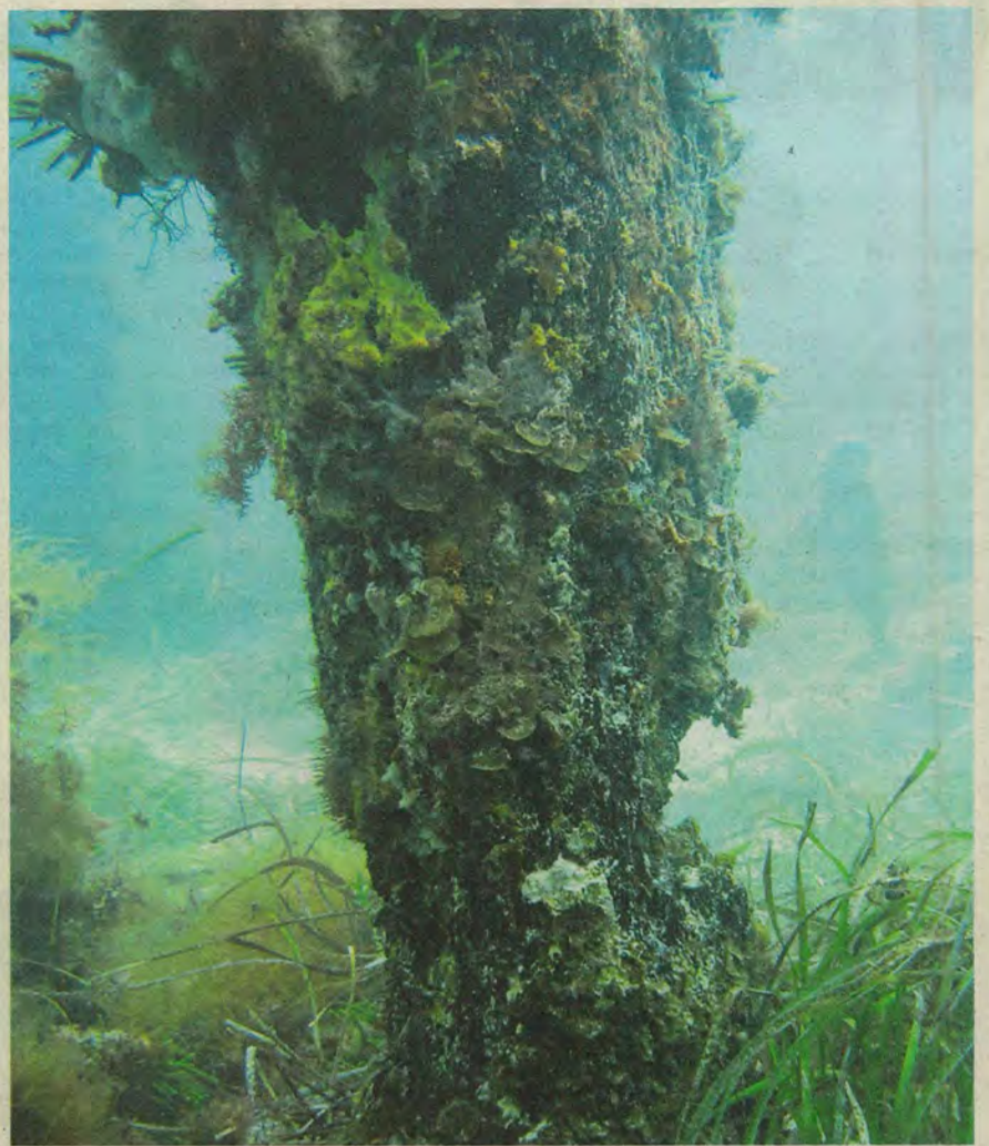
Hanging by a thread: One of the rotting pilons on the tanker jetty.
