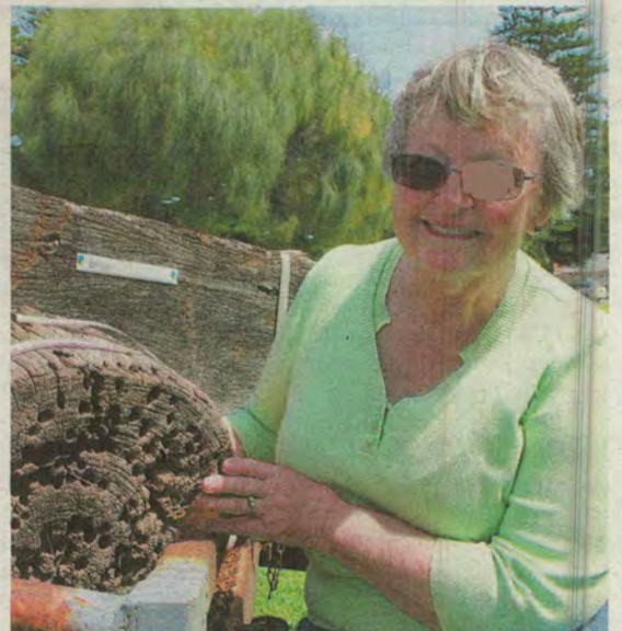
Teredo damage: Marilyn Hart has a look at 1930s pylon that had been attacked by Teredo worms.
