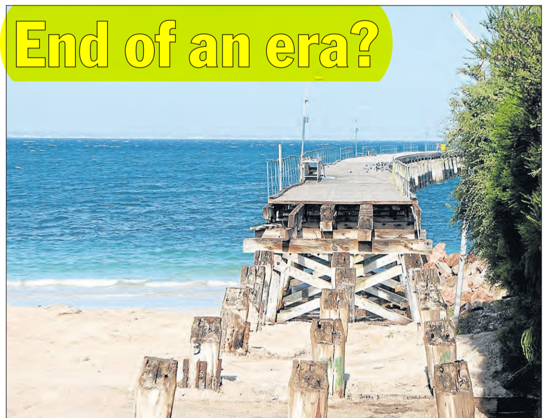
REMOVAL of the first 80 metres of the Esperance Tanker Jetty began on Monday.
