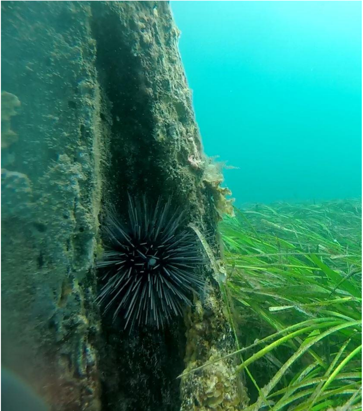
Figure 3-10: 101 North 11/11/15 – Severe section loss at base
