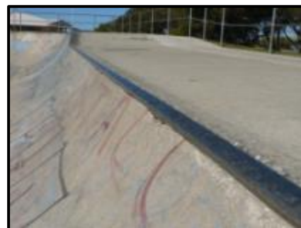
Coping flattened with sharp edges
