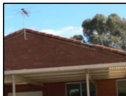
Missing Tiles on Clubhouse
