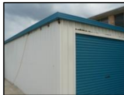
Rusting Storage Shed
