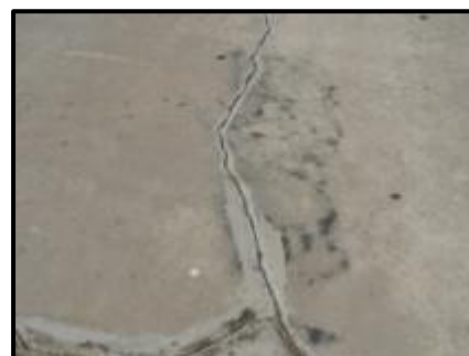
Cracks developing in concrete
