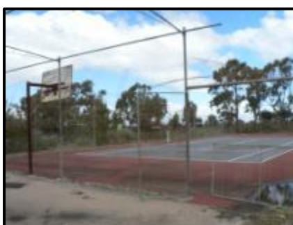
Tennis court in very poor condition
