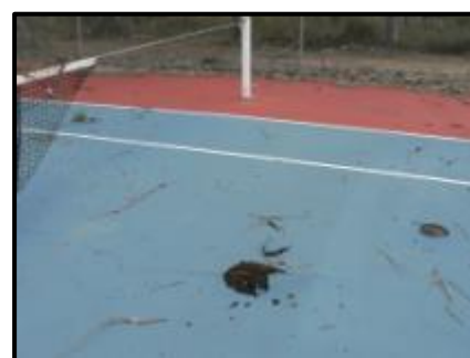
Puff Balls penetrating court surface
