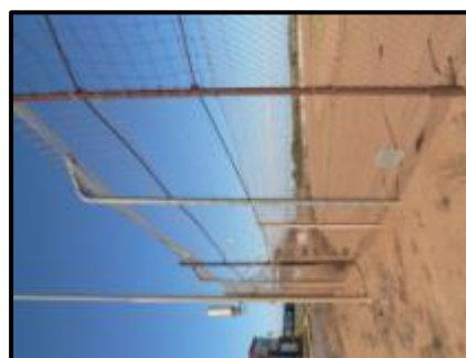
Track fencing showing signs of ageing
